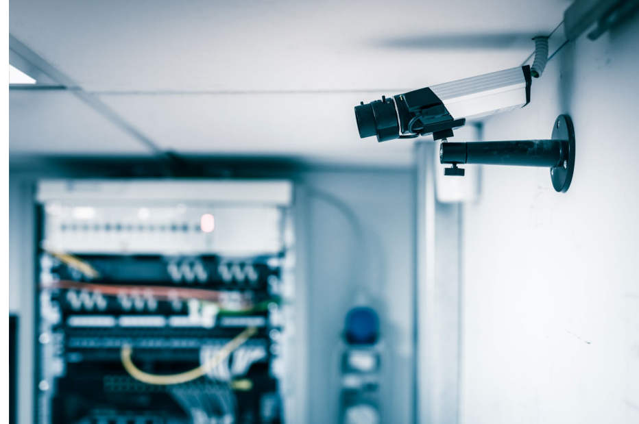
CCTV installed to monitor a server room. (Image by Dario Lo Presti © 123RF.com.)
